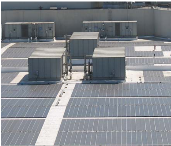
Figure 5: Uni-Solar installation, Long Beach Convention Center.
